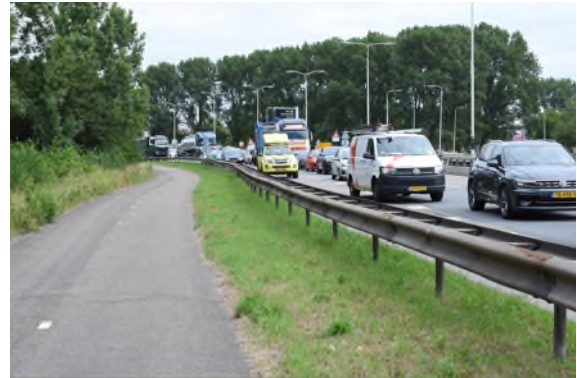
Figure 6. The road is blocked for the safety of labour and traffic users for the critical lifting periods (2 x 15 minutes); View: road side.
