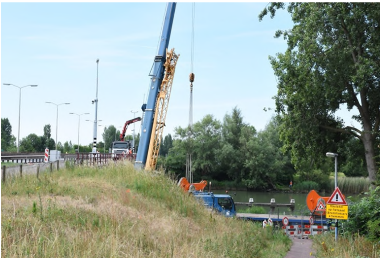
Figure 5. The road is blocked for the safety of labour and traffic users for the critical lifting periods (2 x 15 minutes); View: bridge side.
