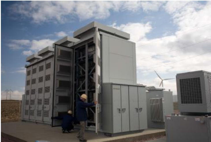
Figure 23: The sodium-sulfur battery connected to the wind farm (source: Himelic & Novacheck, 2011)
