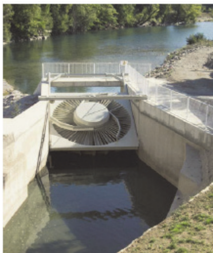
Figure 3-5: Very low head turbine in channel
