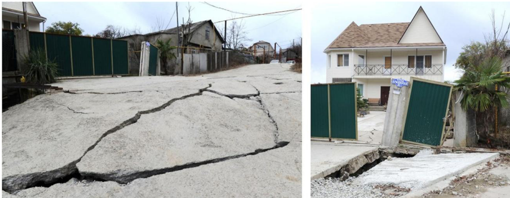
Fig. 7. Damage in the Baranovka village after the landslide movement on 23-24 January 2012.
