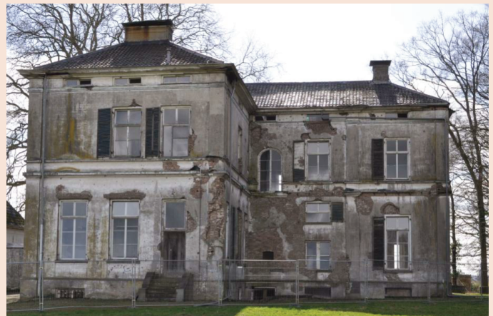
Fig 9. War damage north-east facade House Reuversweerd (BBA, 2019).
