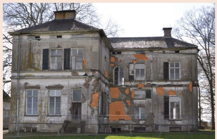
Fig 10. Highlighted immediate repairs of the war damage (BBA, 2019).
