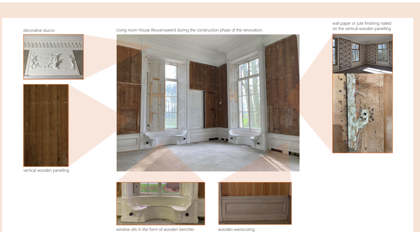
Fig 29. Different finishing layers in House Reuversweerd: decorative stucco, vertical wooden panels with wallpaper, low wooden wainscoting [NL: lambrisering], and window sills in the form of wooden benches.
