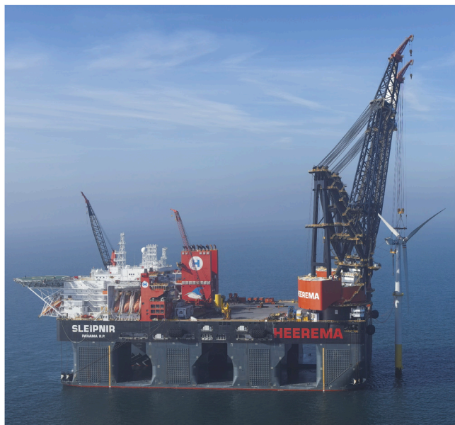
Fig. 1. Semi-submersible crane vessel Sleipnir of Heerema Marine Contractors performing a floating offshore installation of an OWT (DOB-Academy, 2022).
