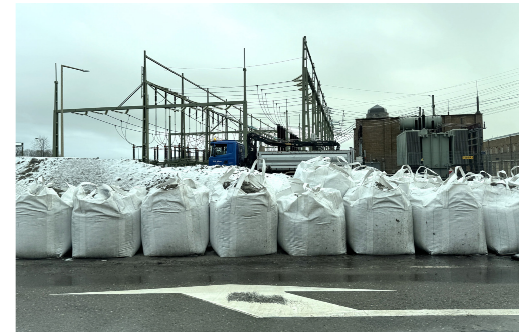
Figure 3.1: Major electrical station serving part of Friesland. Industrially sized sandbags litter the foreground, deployed as protection against flood encroachment.
