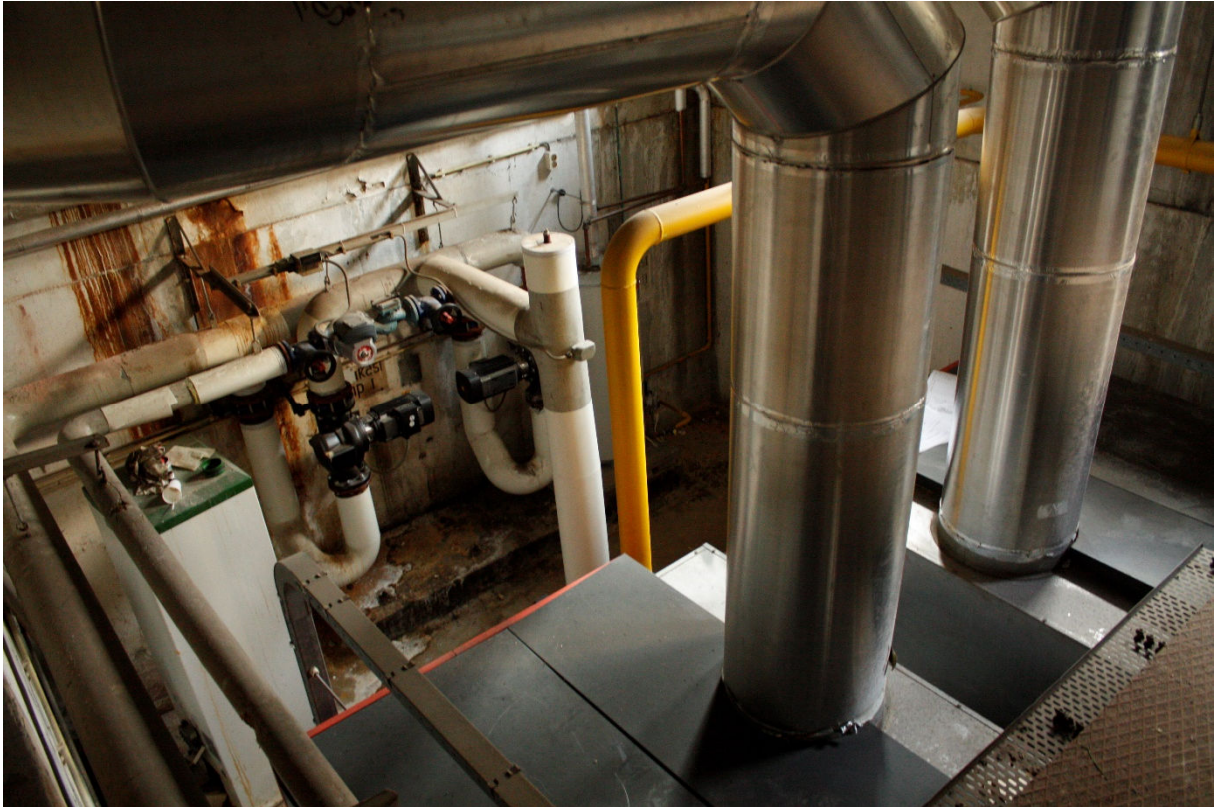
FIGURE 4.29 - THE BASEMENT (1951) HOUSES THE HEATING SYSTEMS FOR THE ENTIRE COMPLEX. PHOTOGRAPH BY STEVEN BEKKERS, 13-2-2015.
