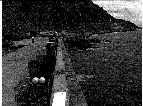
D: Main quay and heavily damaged main breakwater
