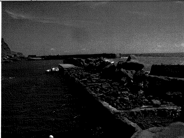
C: Damaged fishery quay
