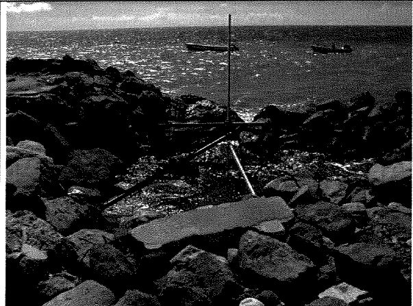
B: Hole in the armour layer of the fishery breakwater
