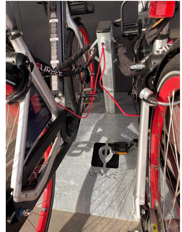
figure 3.6 Stainless steel containers protect chargers from weather influences, red cables draw attention to the chargers
