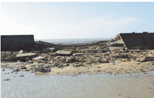
Figure 21: Failure of a flood wall near St.-Martin-de-Ré, on Île de Ré.
