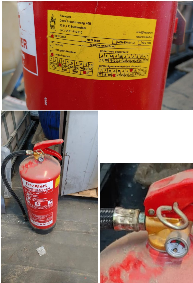
Figure 38: Certificate of fire extinguisher has expired, but the pressure gauge shows enough pressure
