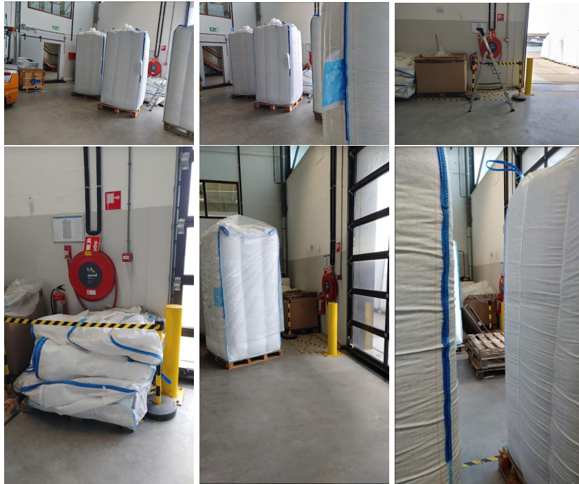
Figure 37: Unreliable access to the fire hose
