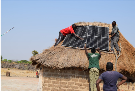
Figure 1.3: Installation of Rooftop PV as part of Solar Home Systems (SHS) in a rural area in Africa [17]
