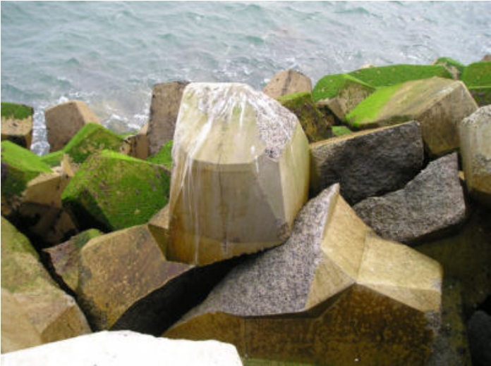
Picture 1-3: Damaged armour units after storm
