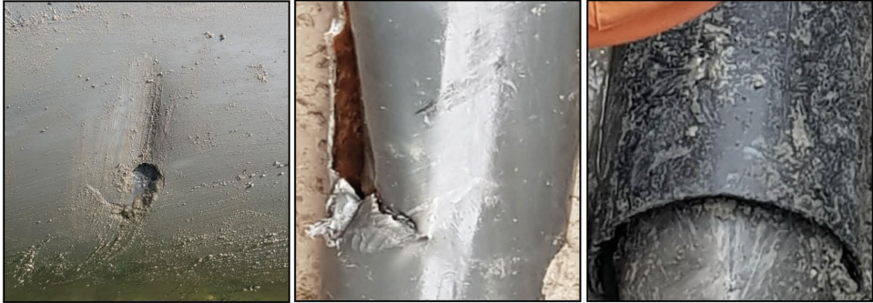
Figure 3.9: In-situ footage after excavation of pipes A-3 (left) and B-2 (middle) with break due to third party impact, and pipe B-3 (right) with crack due to poor installation quality.
