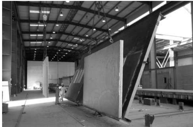
Figure 46 Tilting Table ( https://www.gulfprecast.ae/products/wall-panels/ )
