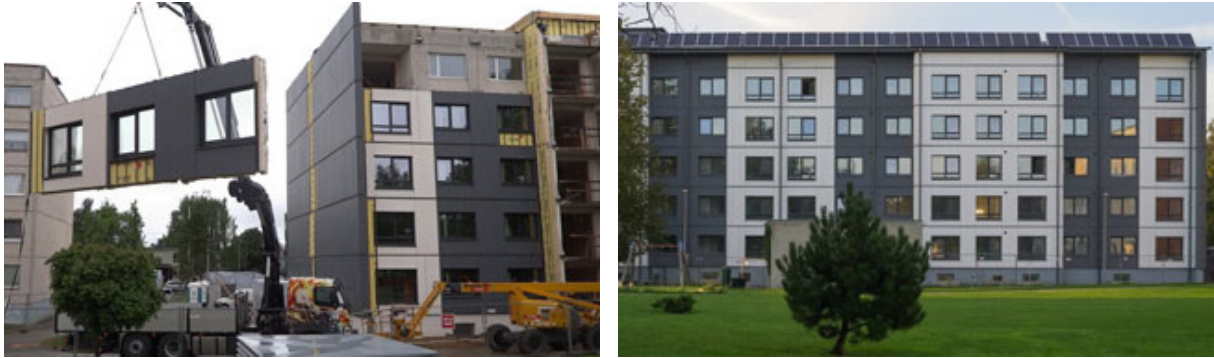
Fig. 2. 5. The installation of prefabricated wall panels on a Soviet-era building in Tallinn, Estonia.
