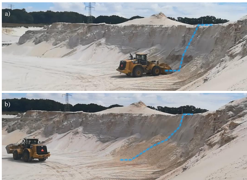
Figure 5.7: a) Slope profile before the last excavation step and assumed geometry used for the numerical simulation (schematic geometry in Figure 5.3 with areaA removed); b) final slope profile, after the induced slope failure.
