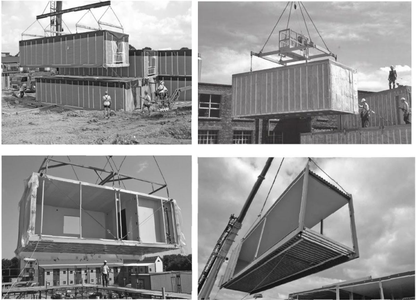
Figure 5.25. Lifting of the modules on construction site (Lawson, M., Ogden, R., Design in modular construction)
