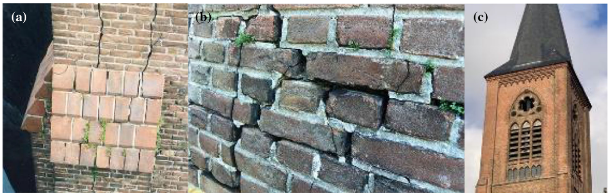
Fig. 19 Cracks in masonry, caused by expansion of bedding mortar, deeper in the wall section, due to formation of thaumasite (a); push out of the pointing is a secondary effect (b); situation several years after repair: no recurrence (c)
