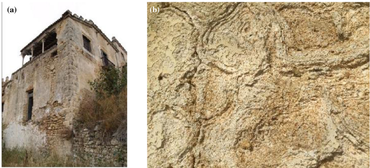
Fig. 27 Valflores Palace in St. Iria da Azoia, Loures, Portugal (a), and Liesegang phenomenon in a rendered façade (b)
