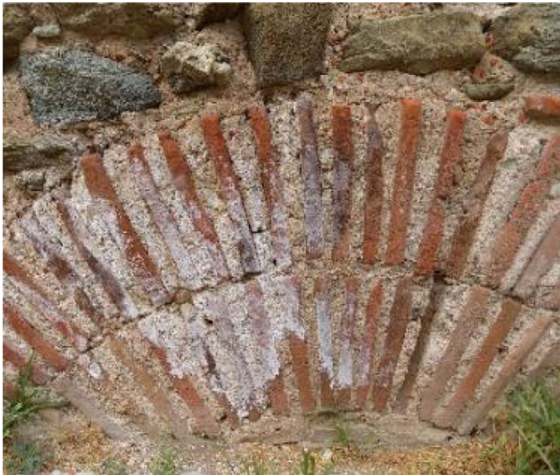
Fig. 31 Efflorescence near to the ground level
