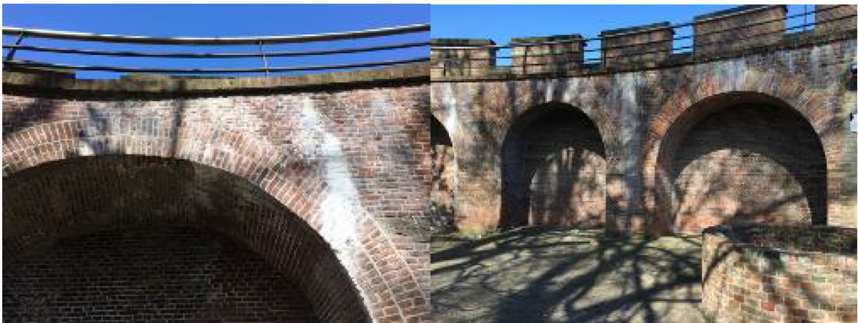
Fig. 16 Lime leaching after repair of historic masonry; see also 4.7
