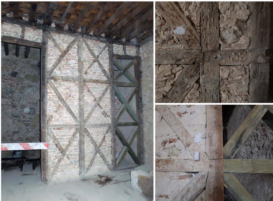
Fig. 2. Internal view of a Pombalino building, Rua dos Fanqueiros , Lisbon (left); original and replaced cross-bracing components (right).
