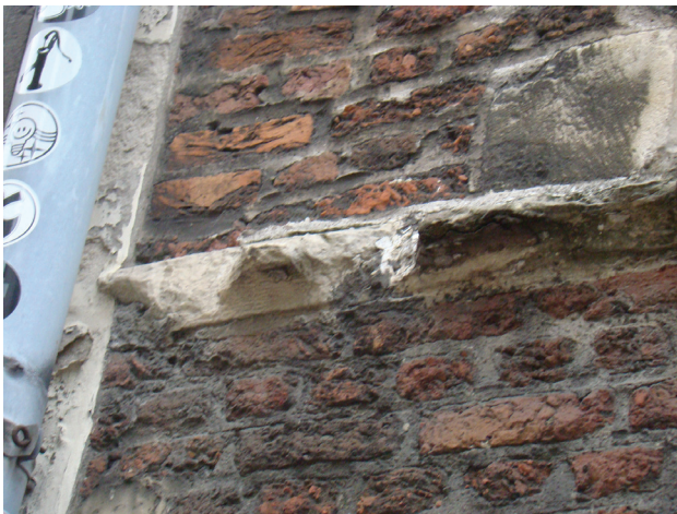
Figure 5: Some parts of the functional elements in limestone are strongly deteriorated.
