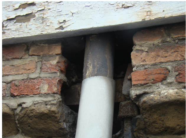
Figure 3: This connection between the gutter and the vertical drainpipe is a delicate point where water infiltrations are likely.
