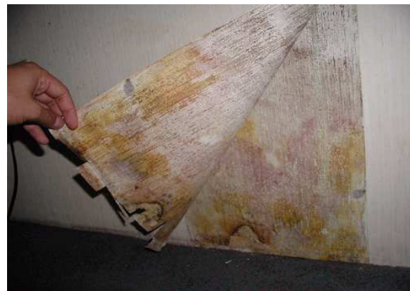
Picture 2-5: Mold due to inwardly driven moisture trapped by the vapor impermeability of the vinyl wall covering; Lit: 46
