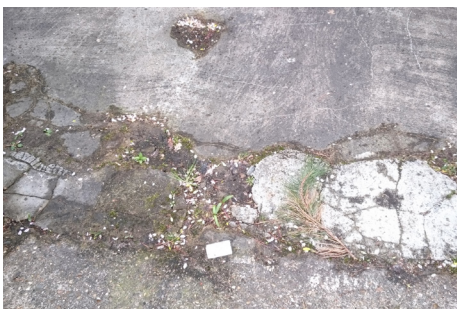
Figure 10: An example of cracked concrete (Franx, 2017).
