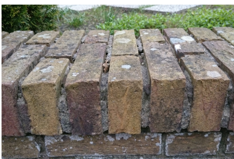
Figure 11: An example of eroded pointing work (Franx, 2017).
