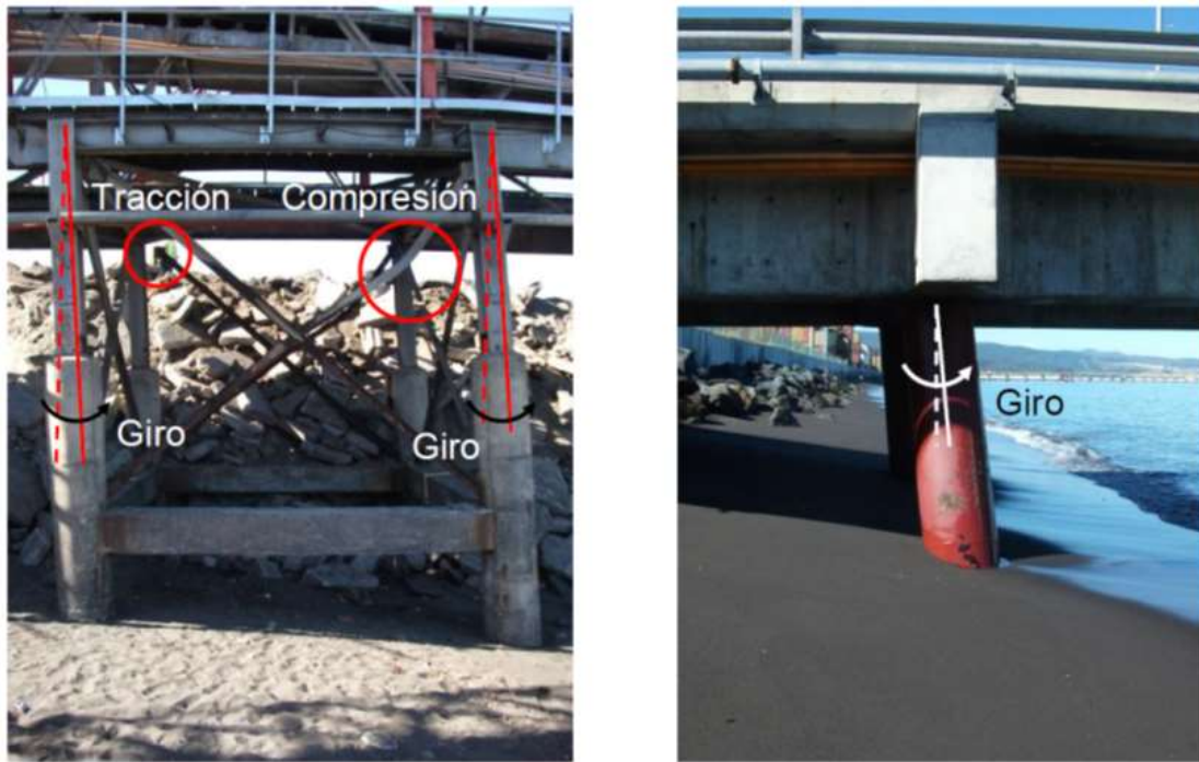
Figure 1-13: System inclination due to lateral spreading at Muelle Jureles (left) and Muelle Coronel Sur (right)
