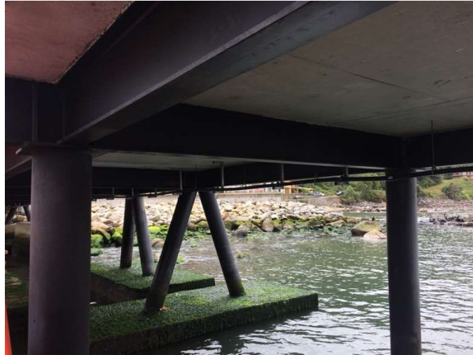
Figure 1-8: Construction detail of the deck, piles, beams and foundation slabs of the Coliumo jetty
