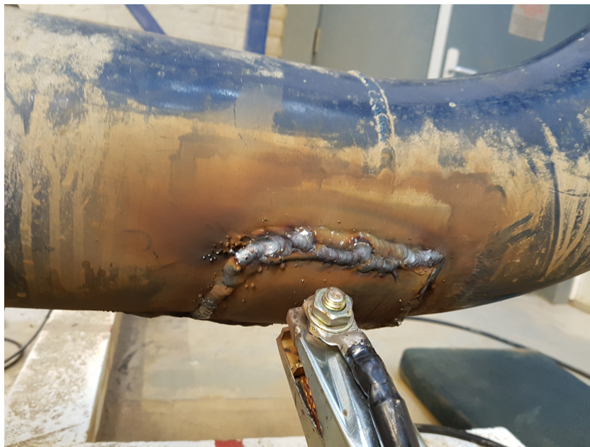
Figure I.8: Worn out descending bend with reinforcements after the weld
