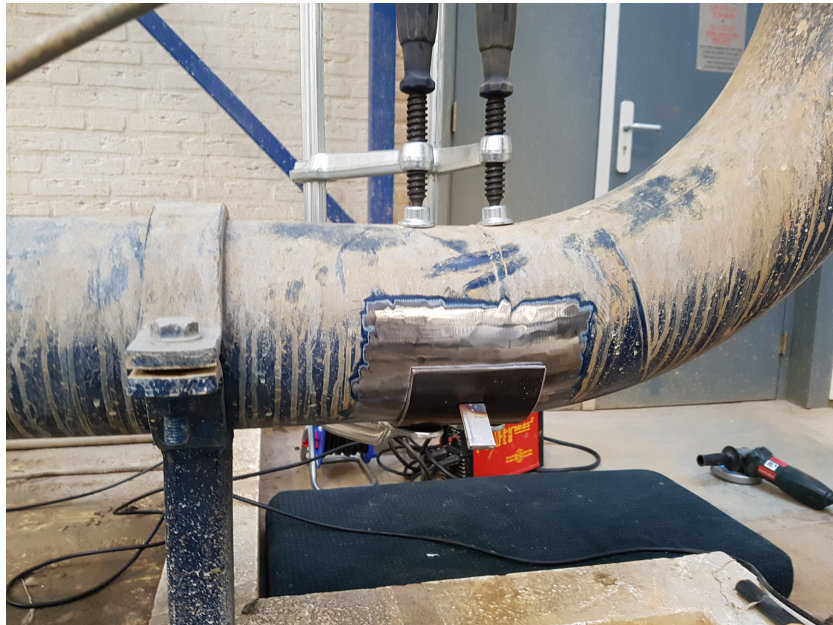
Figure I.7: Worn out descending bend with reinforcements before the weld
