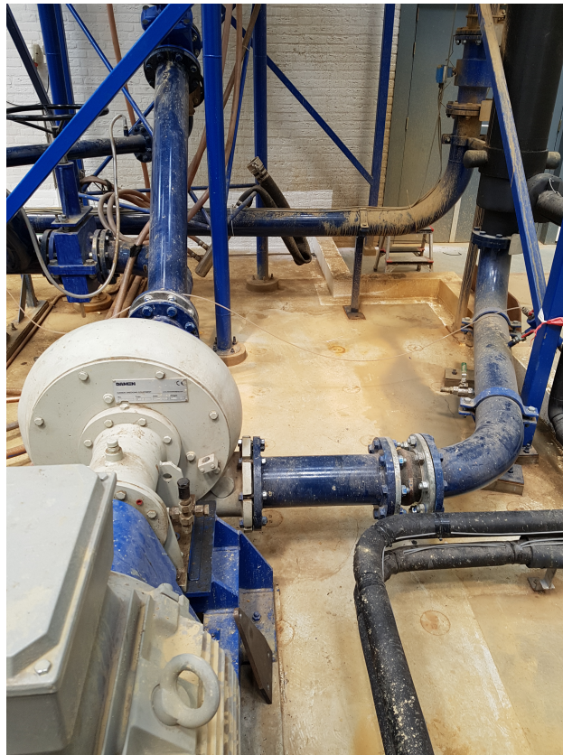
Figure I.1: Back view of the centrifugal pump with discharge pipe
