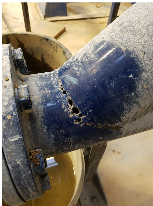
Figure I.9: Worn out weld located on the transition pipe between the storage tank and the suction pipe
