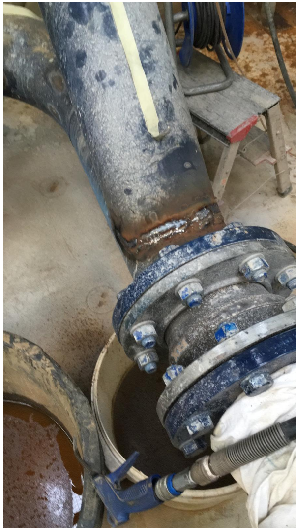
Figure I.10: Repair weld located on the transition pipe between the storage tank and the suction pipe
