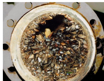
(b) Fouled sea water intake.
