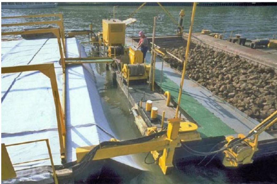
Figure E.19: Geotextile filter placement under water with dedicated equipment. Source: Heibaum (2008)
