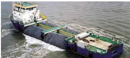
(a) Example of the installation of the scour protection at the Outer locations, indicated by the blue stars in Figure 7.6. Source: Shipshub
