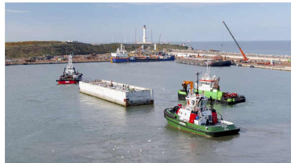
(d) Offloading of the caisson from the Heavy Transport Vessel and towage to the intermediate wet storage.
