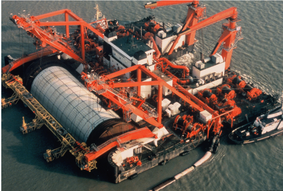
Figure E.18: Specially designed vessel Cardium which has been deployed for the installation of the bed proection for the Easternschelde.
