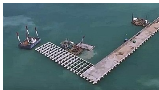
(d) Example of the installation of the caisson units at the Work locations, indicated by the orange stars in Figure 7.6. Source: Dutch Water Sector
