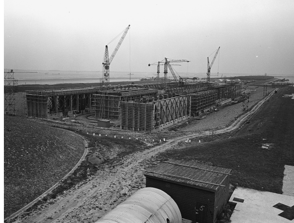
Figure D.3: Temporary construction dock for caissons consists of a polder surrounded by dikes, which can be flooded in a controlled manner to float and thereby enable transportation of the caissons to the desired location. [Image: Rijkswaterstaat]
