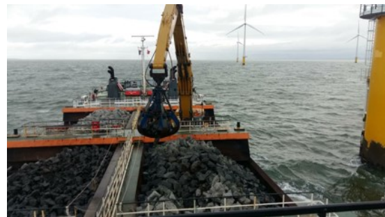
(b) Example of the (more precise) installation of the scour protection at the Outer locations, indicated by the blue stars in Figure 7.6. Source: Van Tunen
