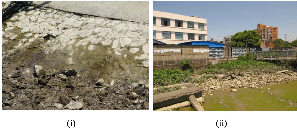
Fig.2. 20 Field observations on the vulnerability of floodwall along the Huangpu River in 2013: (i) leakage and (ii) the close connection between flood defence system and buildings
