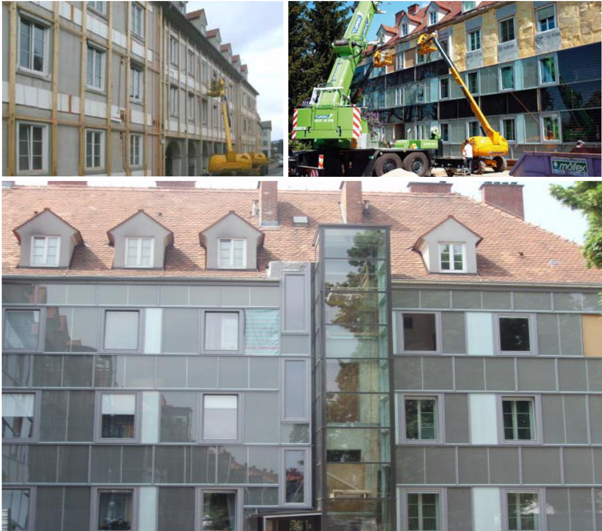
Figure 4.8: Heat pipes are attached to the existing facade first (Top left) before being covered with rockwool and afterwards the new facade (Top right). The facades facing South were integrated with solar thermal collectors. The rest only featured solar combs. (Bottom)
