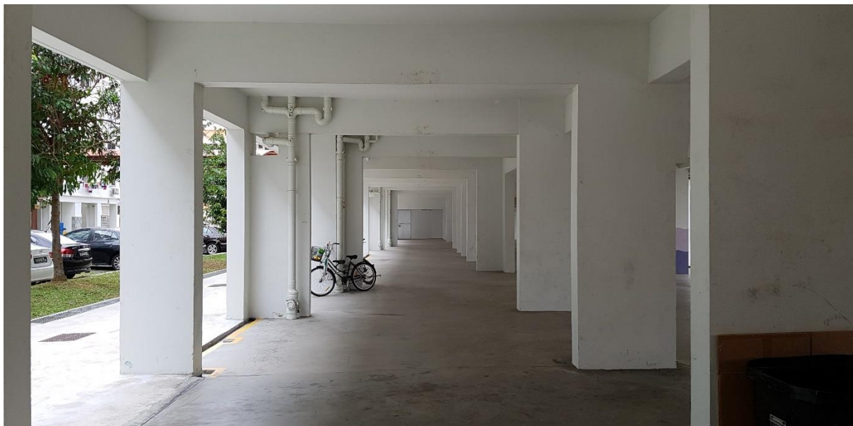
Figure 4.31: The ground floor of the building. Only structural columns occupy the space.
