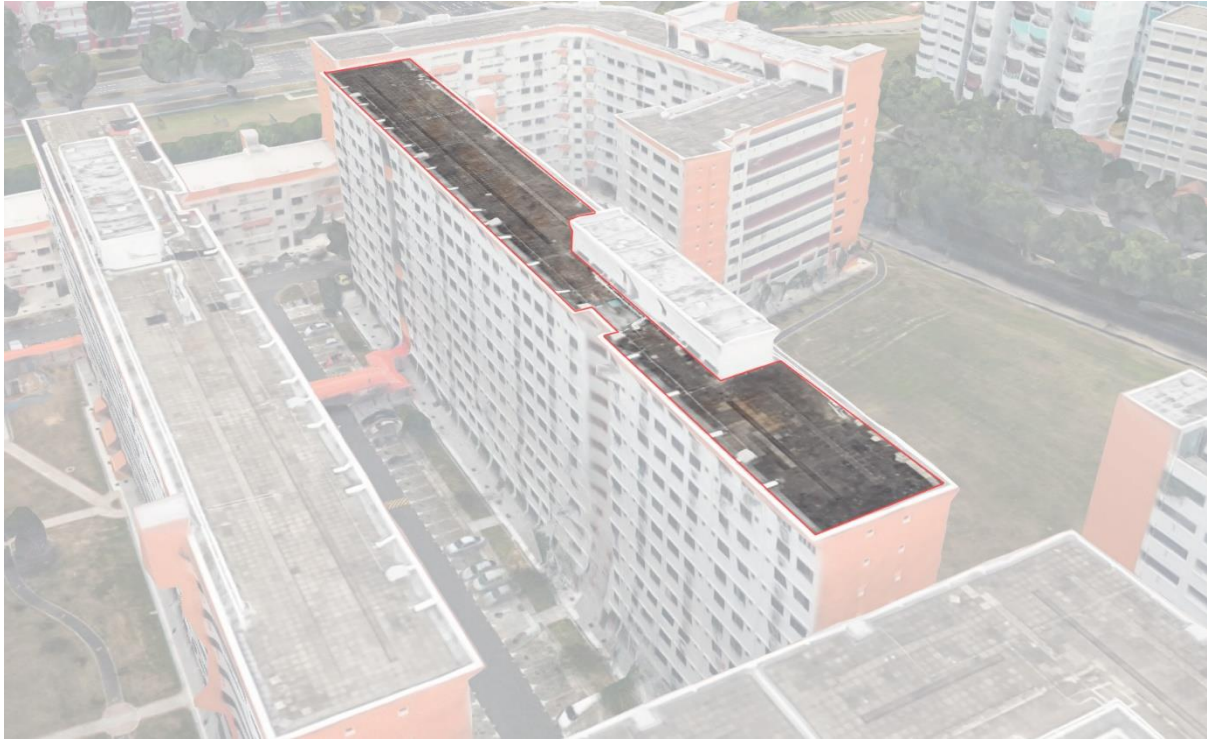
Figure 4.30: A Google Maps image of the roof of the building from Northwest direction.
