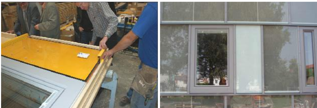
Figure 4.7: The ventilation ducts are integrated within the facade module (Left) beside the window, where an opaque covering is placed over the supply and exhaust ducts (Right).
