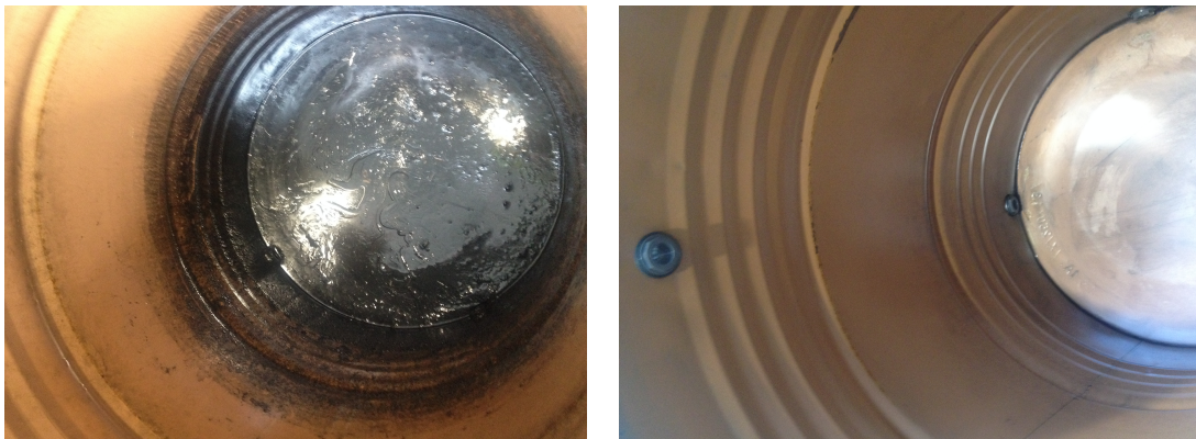
Figure 4.10: Photographs of the inside of the separation vessel. Left: Vessel after all fluids have been removed. The black residue are dead bacteria mixed with oil. Right: Clean inside of the separation vessel.
