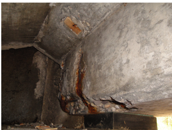
(a) Spalling concrete and corrosion damage to the beam head
