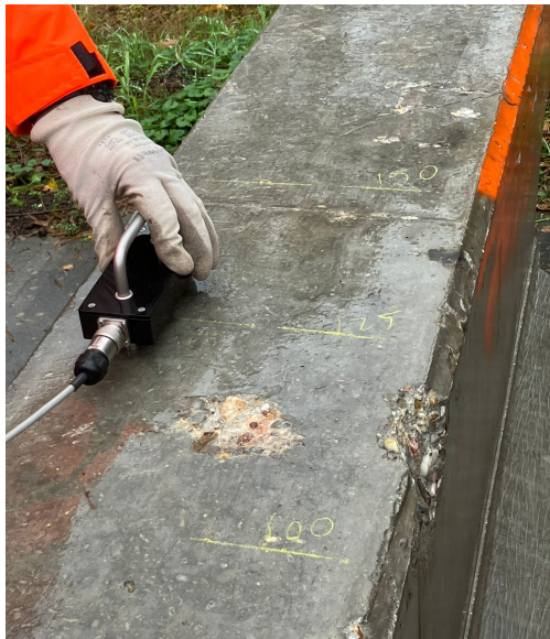
(c) Minor surface defects on beam L2. Markings for the measurement grid can be seen in yellow.
