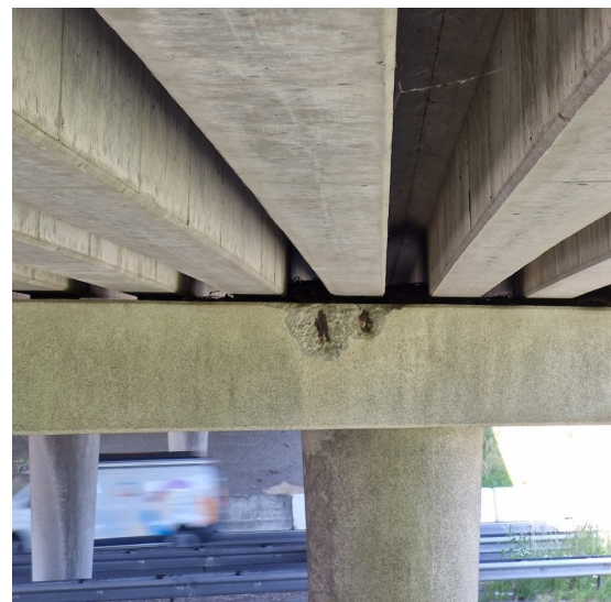
(d) Exposed reinforcement at the right side of support beam 4
