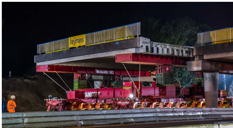
Figure 3.15: A SPMT truck lifting one of two inner spans to be transported for later research. Photo by Hans Broekhuizen [53]
