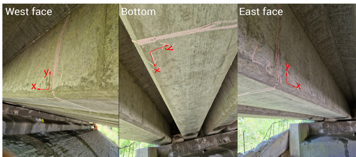
Figure C.1: The local axis for the Profometer measurements.
