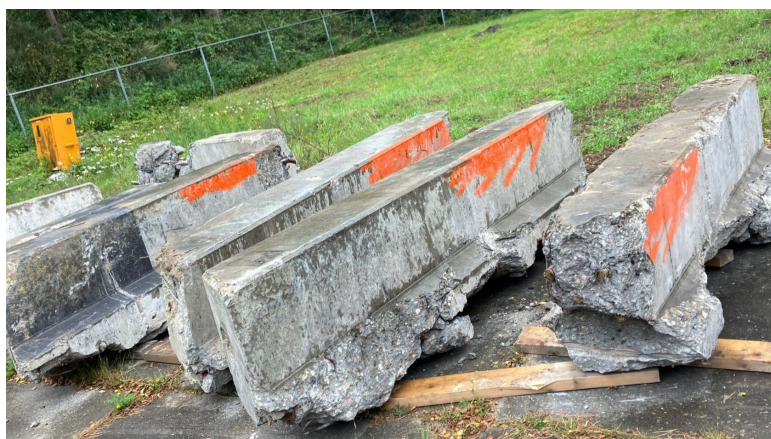
Figure 3.16: The harvested beam heads from the Ardeweg Viaduct at the Rijkswaterstaat location in Wolfheze.
