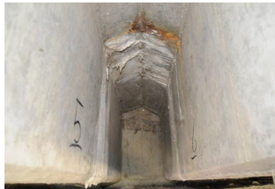
(b) Visible leakage between the beam heads of beam 5 and 6 at STP5
