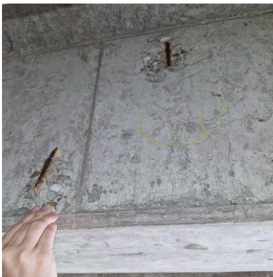
(a) Minor corrosion damage on the side of beam 21
