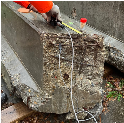
(a) Absent concrete cover at the end of the beam head of L13 with exposed reinforcements. Resistivity test is being performed.
