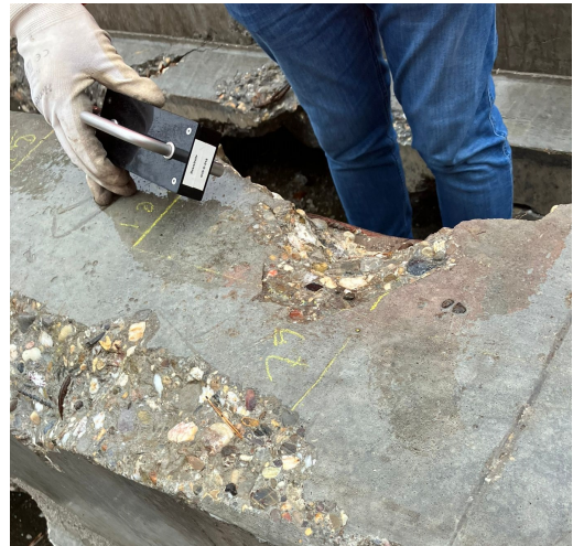
(b) Broken edges and surface damage at the top surface of beam L23, making measurements at this location difficult.
