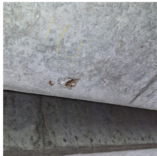
(b) Minor corrosion damage on the bottom of beam 14
