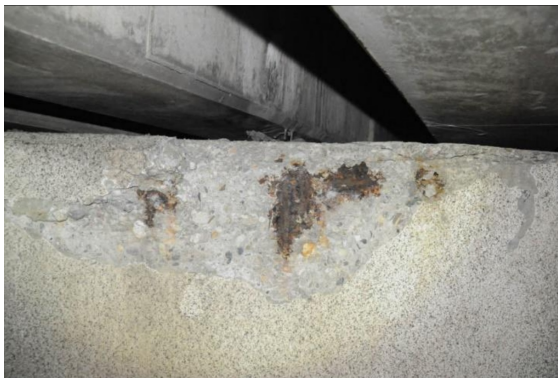
(a) Damaged concrete corner at support beam 4 (STP4) with signs of corrosion
