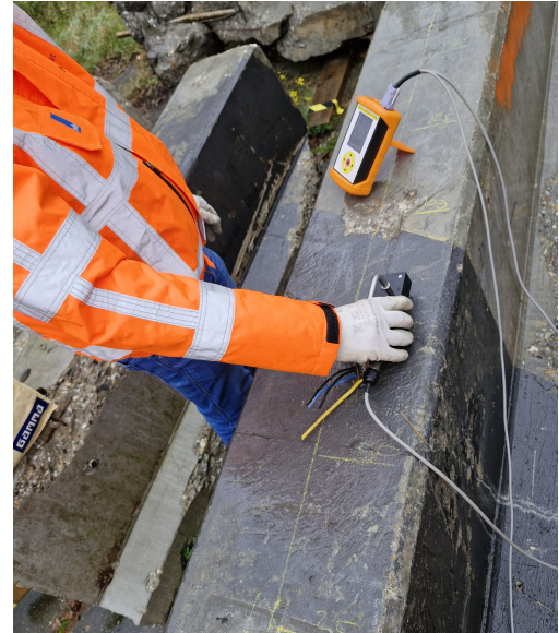
(d) Resistivity measurement being performed with the Gecor-10 on the cathodic protection coating on beam L17.
