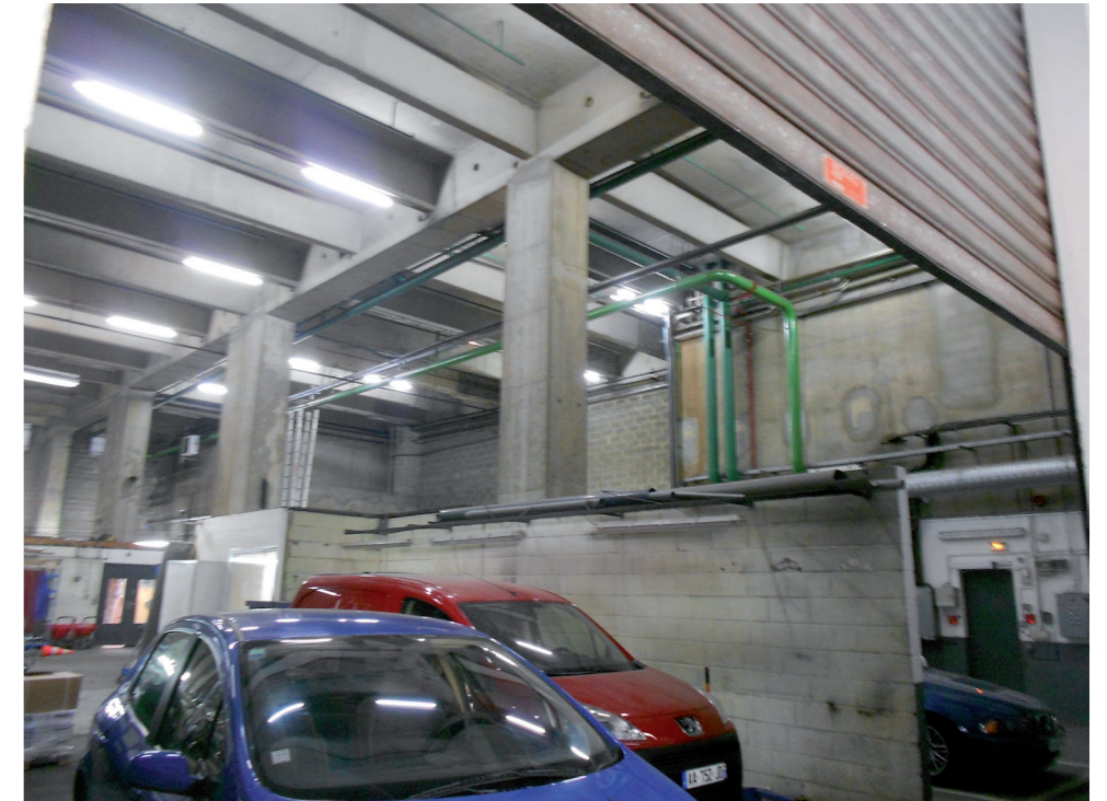
Visible cement to close the joints between the separate prefab and in situ construction elements on the ground floor.
