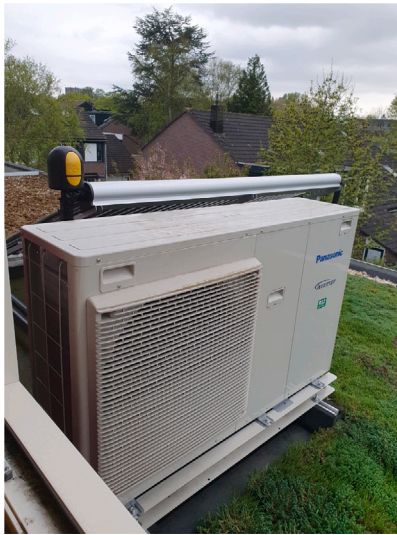
Fig. 2. View from the roof of the retrofitted house. From left to right: solar boiler, heat pump and sedum roof cover (picture by first author).
