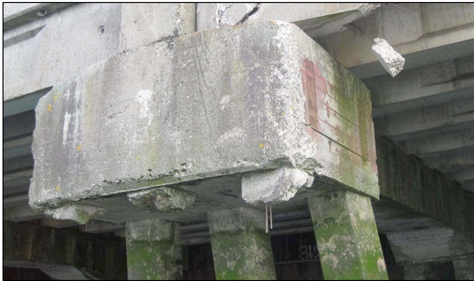
Figure 5. Photo of south section, 3 piles missing underneath single trestle
