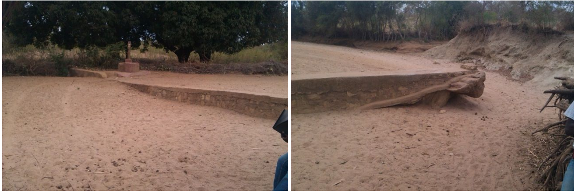
Figure A.33 Sand dam 25 (left) with eroded wing wall (right)
