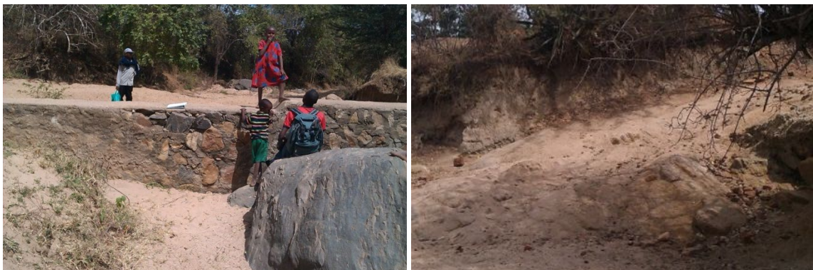
Figure A.11 Sand dam 7 (left) with eroded wing wall (right)
