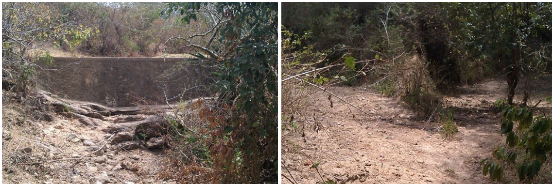
Figure A.37 Left: Eroded riverbed downstream of sand dam I; Right: Junction of the streams of the two main sources
