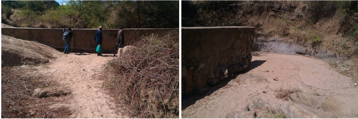
Figure A.9 Sand dam 5 (left) with eroded wing wall (right)
