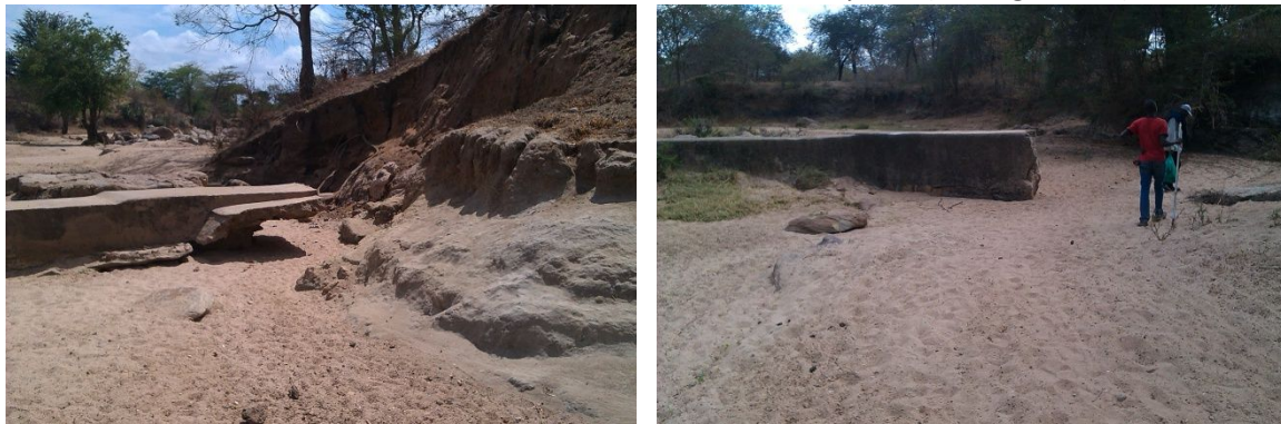
Figure A.2 Failed sand dams (left: sand dam 21, right: sand dam 9)
