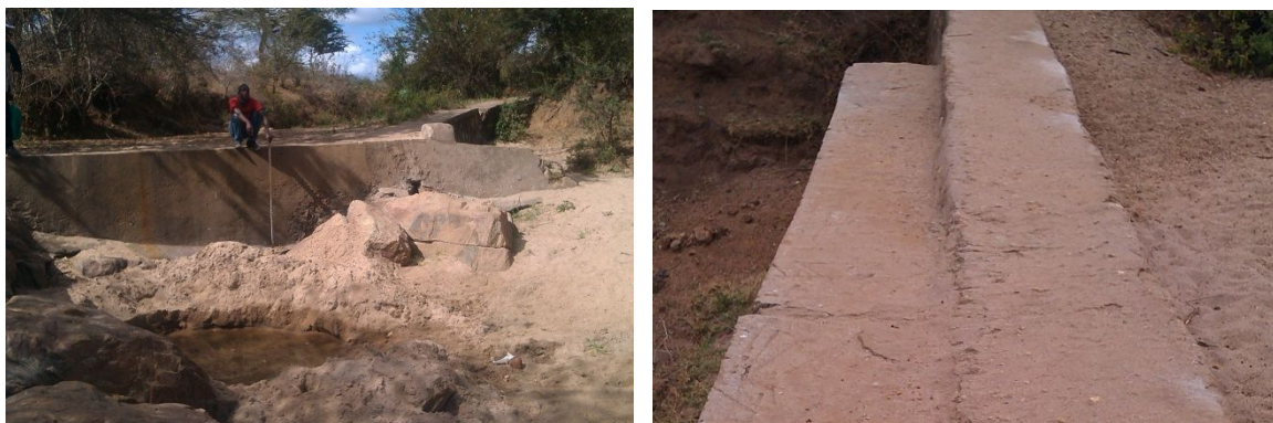
Figure A.3 Repaired sand dams (left: sand dam 8, right sand dam VI)
