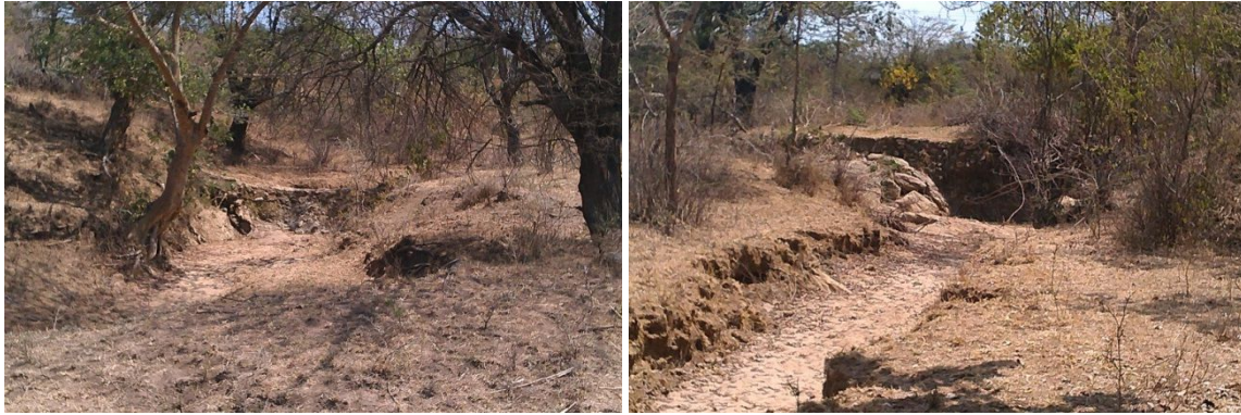
Figure A.20 First (left) and third sand dam (right) of a cascade of three private sand dams in a tributary
