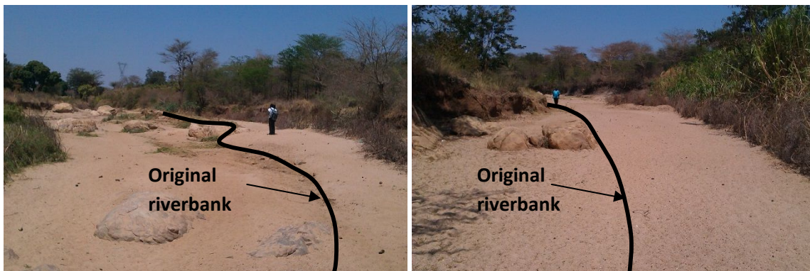
Figure A.46 Eroded riverbanks downstream of sand dam 16
