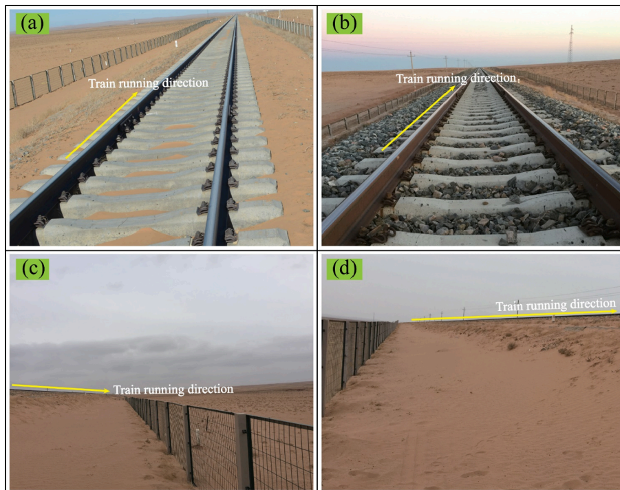
Fig. 2. Site conditions: (a) sandy section, (b) clean section, (c) Front view of train operation direction, (d) Back view of train operation direction.
