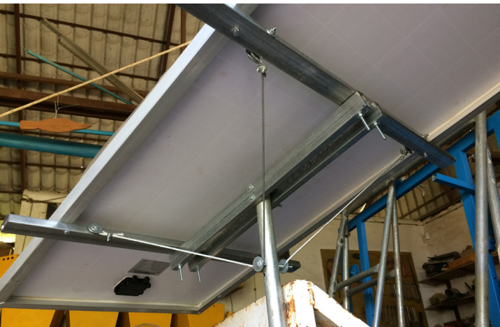
figure 90. The cables should be professionally connected
