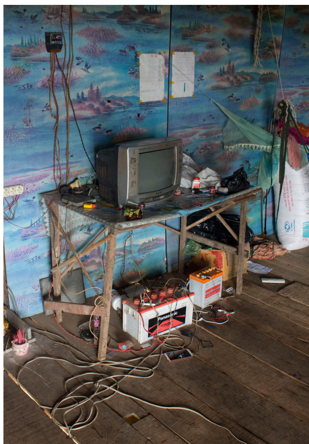
figure 15. Self-installed solar energy inside
