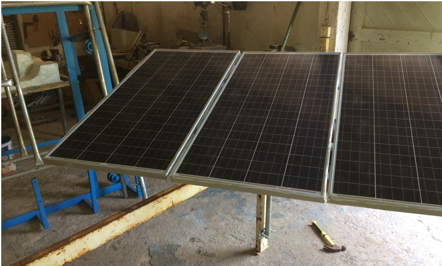
figure 95. Three large solar panels mounted on the mounting pole (SA workshop)
