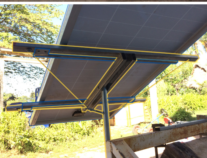
figure 94. Expansion arms made from galvanized steel
