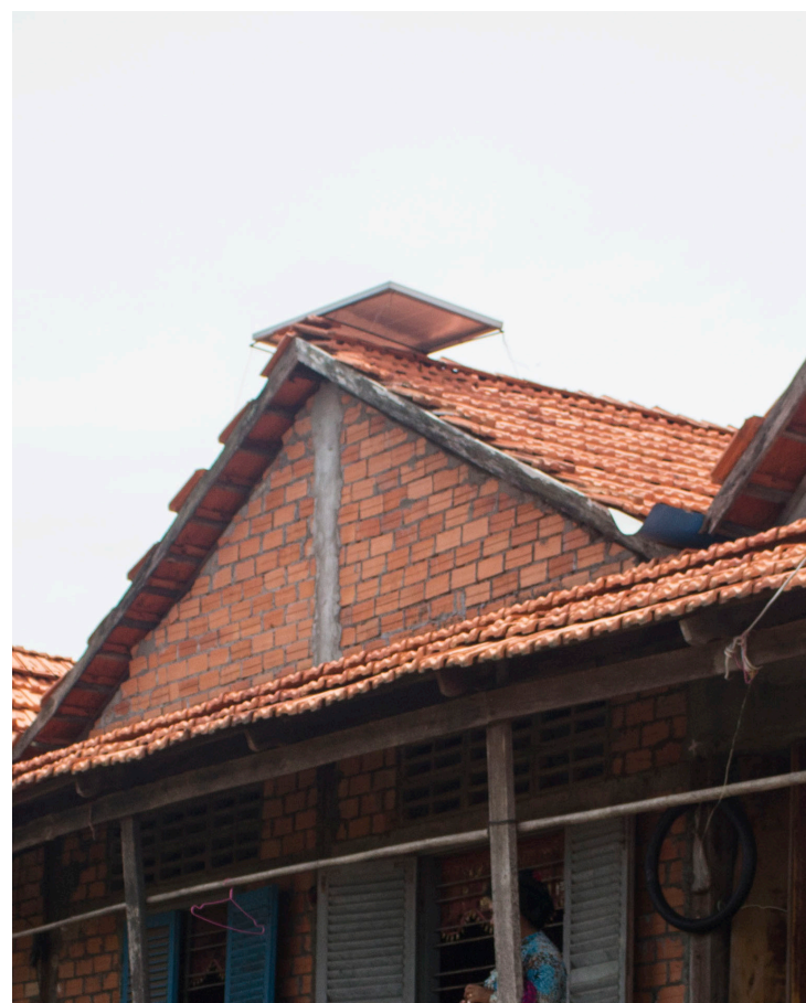
figure 16. Self-installed solar panel
