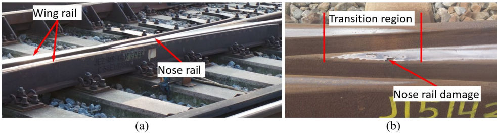
Figure 1.2. A 1:9 cast manganese steel crossing: (a) View of a wing rail and crossing nose rail; (b) Crossing nose rail damage in the transition region.
