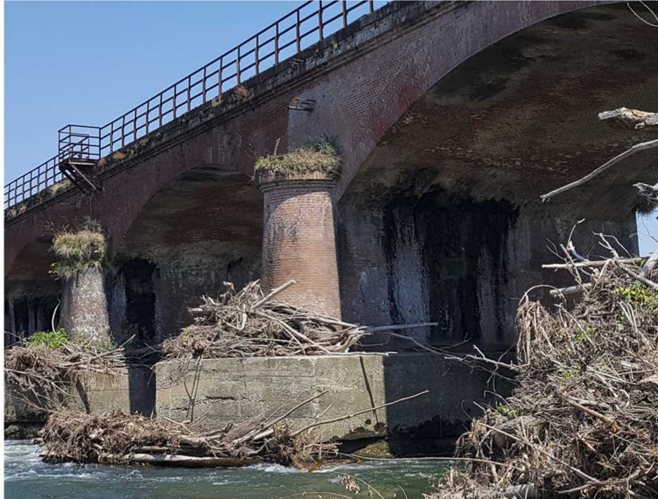
Figure 5.3: An example of debris accumulation after flooding [154]
