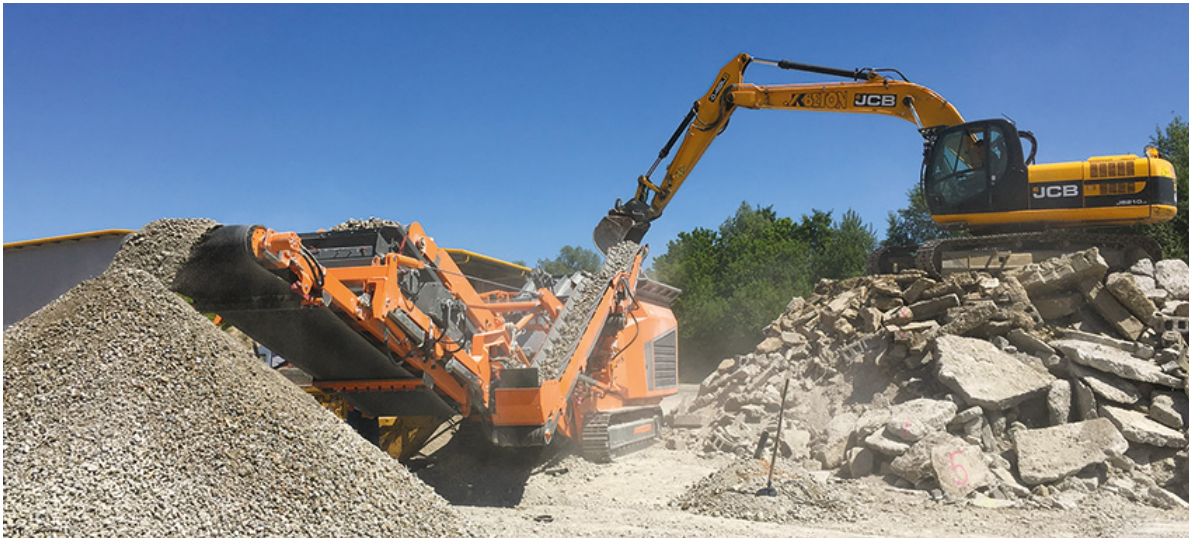
Figure 2.5: Mobile C&DW recycling plant (ROCKSTER®)
