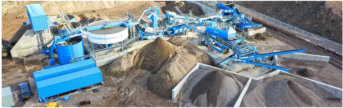
Figure 2.6: Example of a wet concrete recycling plant (CDE ® , 2022)
