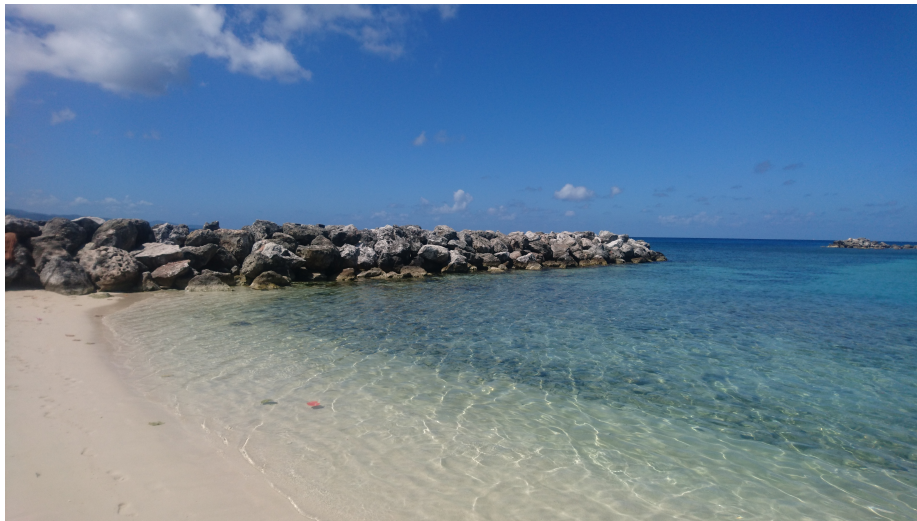
Figure A.7: Present state of groyne 2.
