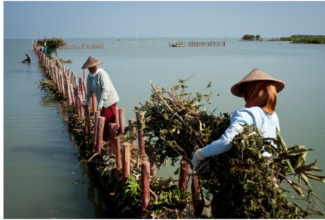
Figure 4.10: Building with Nature in Java, Indonesia. Natural materials are used to create permeable dams to prevent coastal erosion (See Appendix B).
