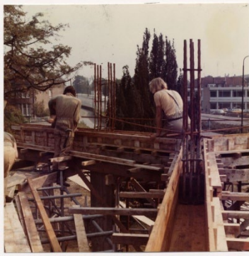
Heemkundekring Helmont (n.d.). Laying of the floor beams [Photo]. Retrieved April 2 nd 2025, from https://indebuurt.nl/helmond/genieten-van/toen-in/toen-in-helmond-zo-zag-de-bouw-van-de-kubuswoningen-eruit~151569/#slide-2
