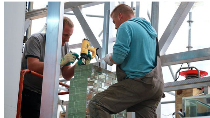
FIGURE 59: Figure showing installation of facade of solid blocks with adhesives in Crystal house (Archdaily, 2016)
