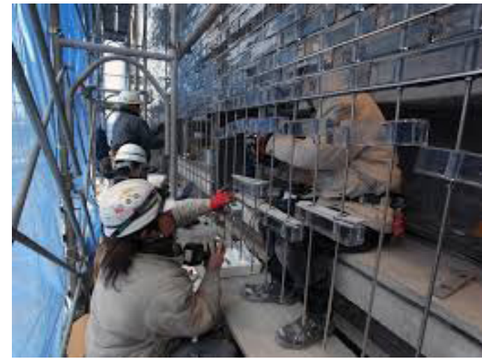
FIGURE 48: Figure showing installation of facade of solid blocks with metal support in Optical house (Archdaily, 2020)
