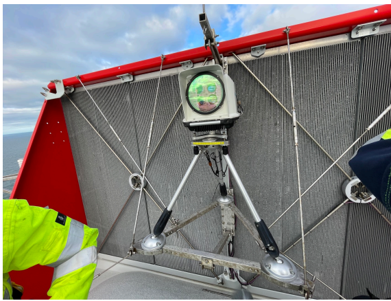
(a) The WindCube Nacelle Lidar during installation.
