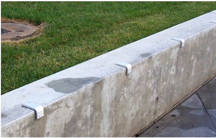
Fig. 4.21 - Grind-prevention on a concrete barrier, 2006. Creating durable grindable surfaces in public space could prove more cost-effective in the long run. Photograph by Wikimedia user Mboverload.
