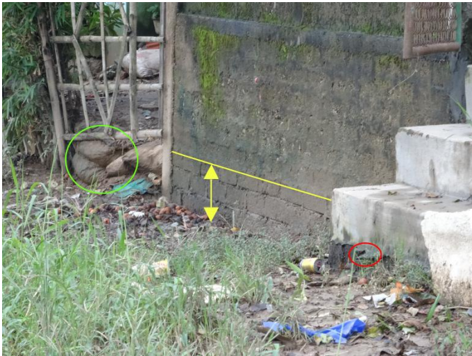
FIGURE 15: EROSION ALONG THE WALL (YELLOW) AND UNDER THE STAIRS (RED) ALSO SANDBAGS ARE STILL LOCATED IN FRONT OF THE GARDEN (GREEN)
