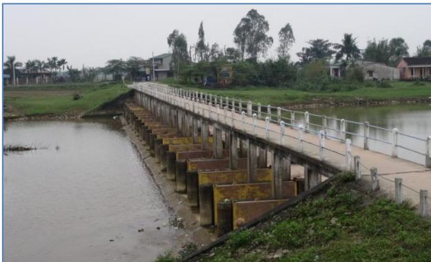
FIGURE 146: A WEIR LOCATED ALONG ONE OF THE TRIBUTARIE OF THE HUONG RIVER
