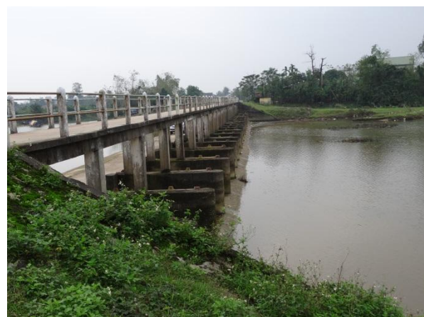
FIGURE 100: AN EXAMPLE OF A CONTROL STRUCTURE THAT LIMITS SALINE WATER FLOW INTO THE BASIN
