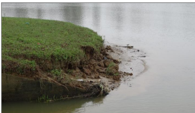
FIGURE 147: EROSION NEAR THE WEIR
