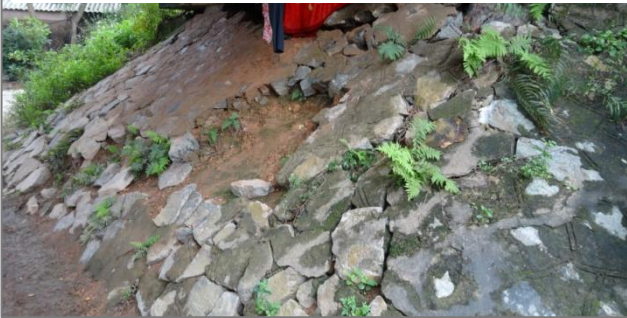
FIGURE 139: EROSION SPOT AT THE ABUTMENT OF A BRIDGE
