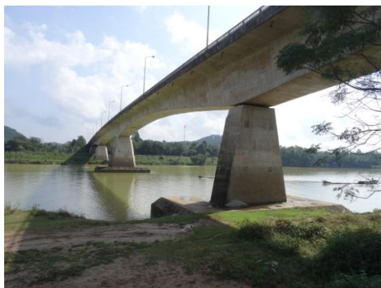
FIGURE 68: THE CURRENT BRIDGE OF THE MAIN ROAD WHICH IS LOCATED INSIDE LAKE HUE
