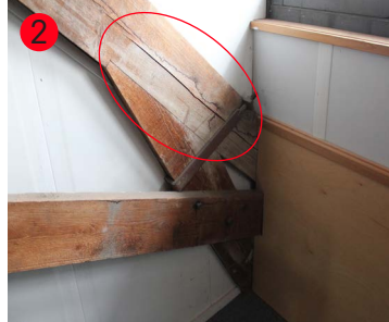
Image 161 Splits on wooden beam
