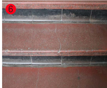
Image 165 Cracks on threads
