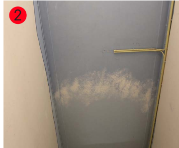
Image 172 Damage on ceiling
