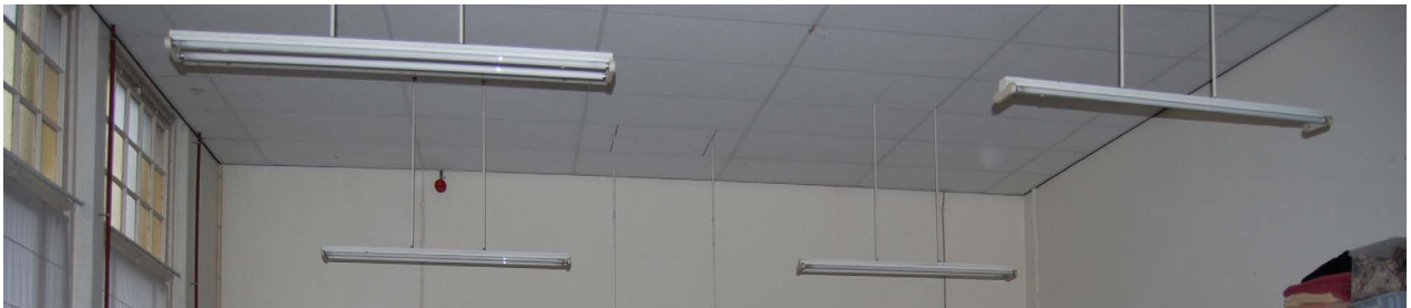
Image 188 Lowered fluorescent tubes in St. Anna
