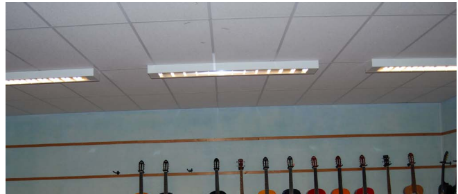
Image 187 Fluorescent tube lighting in the extension
