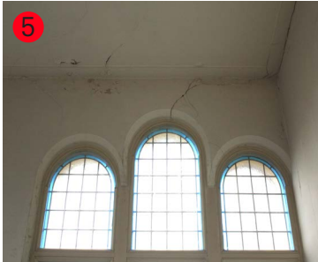
Image 175 Cracks on west facade
