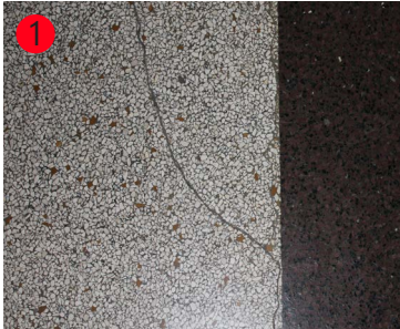
Image 171 Cracks in terrazzo flooring
