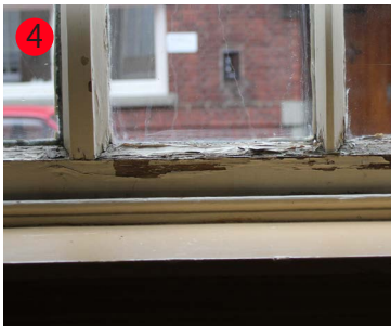
Image 174 Damage on window frame
