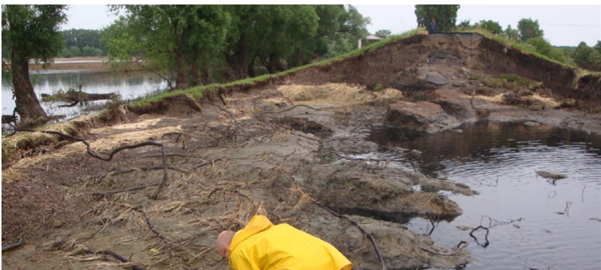
Figure 2.7. Photo of the cross-section of the breached levee (Grubert, 2013a)
