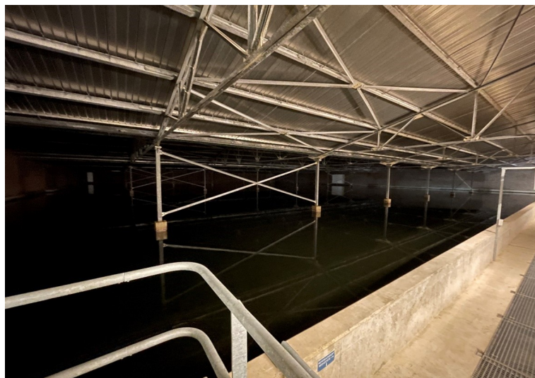
Figure 5: Slow sand filter still in production (mature bed)
